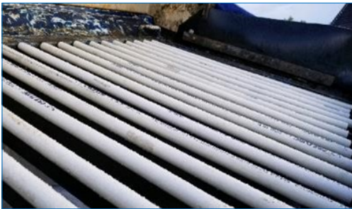
PVC pipe or a cut hose placed over conventional straight slit grates can be used as a "quick solution" for a rounded grate system
