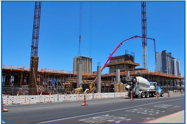
Figure 8. 601 N. Central Phoenix, a mid-rise building project, Phoenix, Arizona days) to this project. It should be mentioned that a special 3/8" basalt aggregate was used in the
