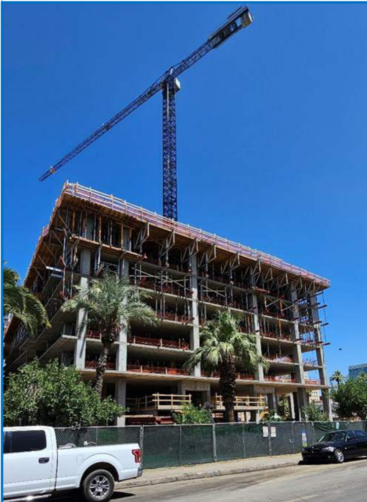
Figure 7. McKinley Green multi-family, high-rise building project, Phoenix, Arizona. Phoenix, Arizona. CalPortland is supplying a variety of high strength SCC (8, 10, and 12 ksi at 28
